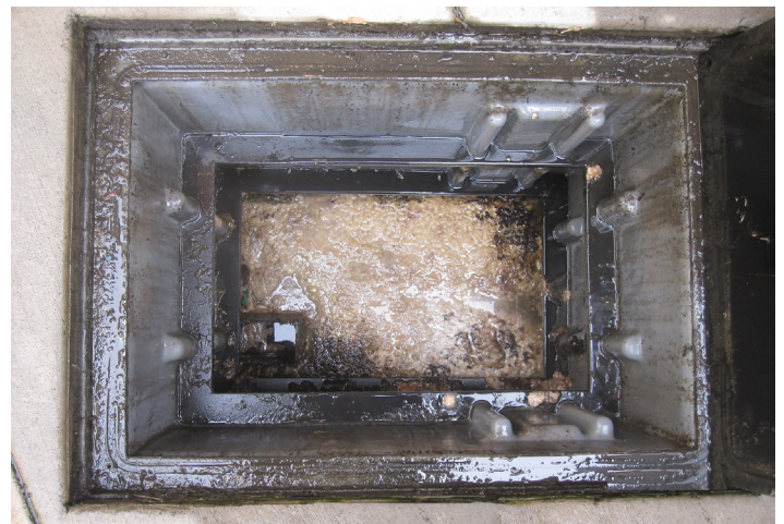
Interceptor operating correctly.
