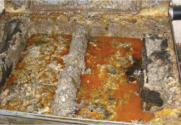
Interceptor pumped out - NOT cleaned to standards.
