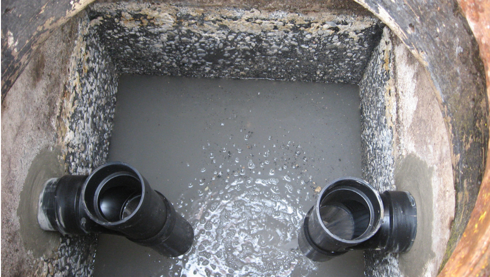
A well-cleaned and compliant grease interceptor.
